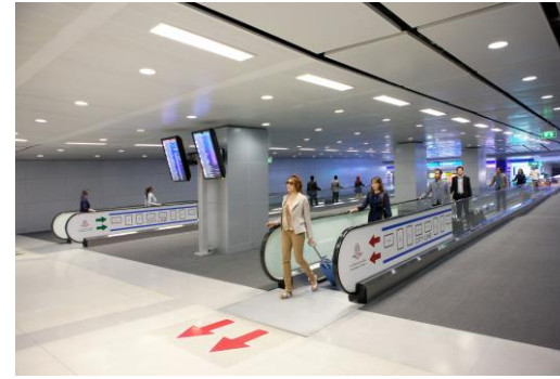
Suvarnabhumi Airport Rail Link 140 units
